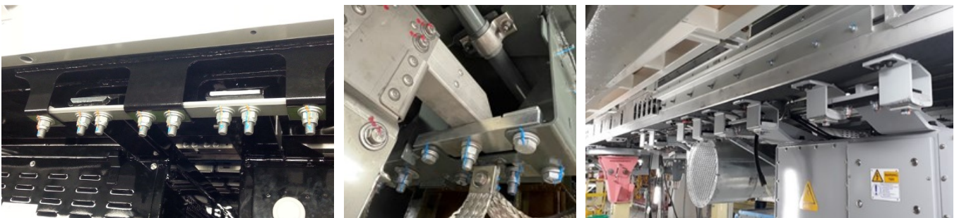
Figure 4: « Positive » equipment mounting on metro platform
